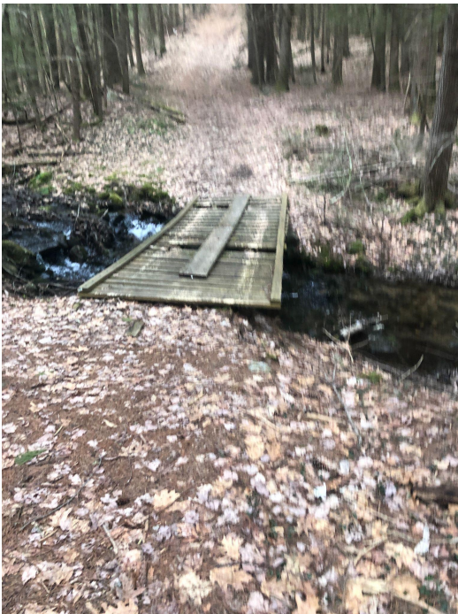
Photo 29. Bridge in poor condition.
