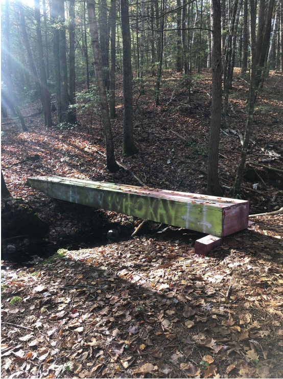
Photo 5. Graffiti on bridge.
