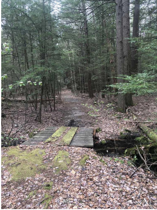
Photo 21. Bridge in poor condition.
