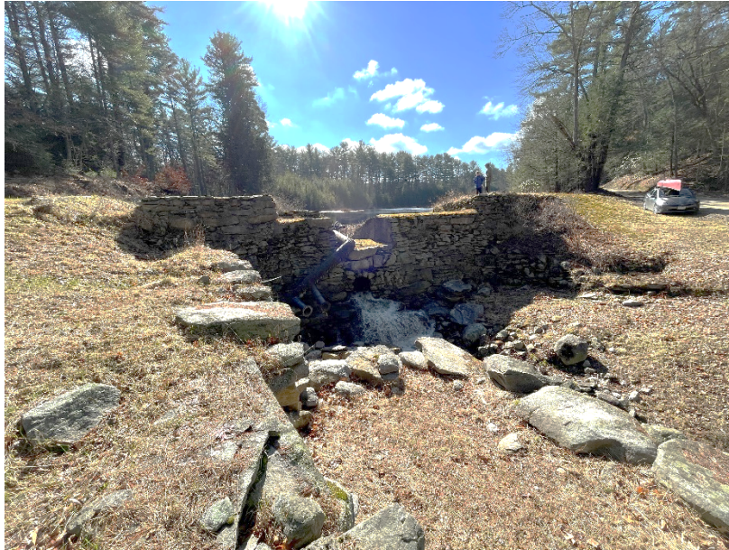
Photo 1. Overview of the dam facing upstream from the downstream right upper masonry wall
