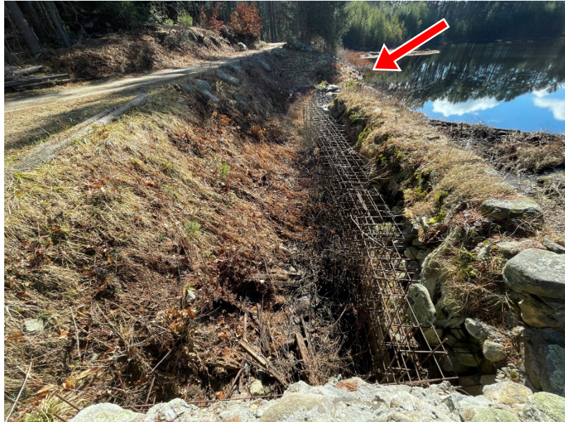
Photo 7. Overview of the excavated void space behind the right dam wall facing upstream; note location of potential overtopping during high flow conditions into the excavated void space
