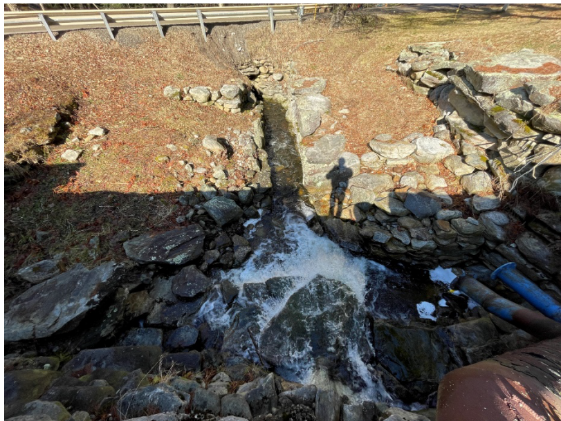
Photo 6. Overview of the downstream channel and downstream Montague Road culvert facing downstream from the spillway
