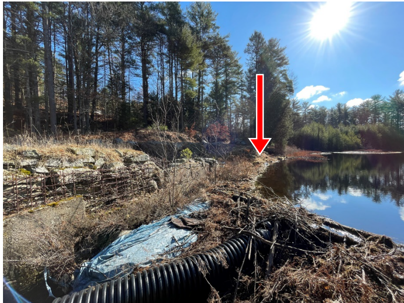
Photo 5. Overview of the beaver dam from the spillway upstream end of the spillway facing; note location of potential overtopping during high flow conditions into the excavated void space
