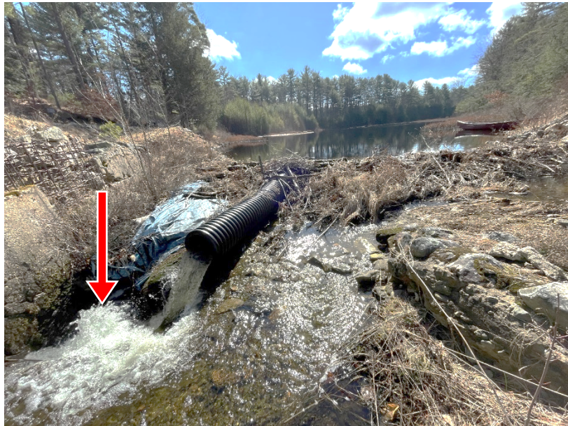
Photo 3. Overview of the beaver dam from the dam primary spillway facing upstream; note where the beaver deceiver outlet discharges into the low-level outlet pipe
