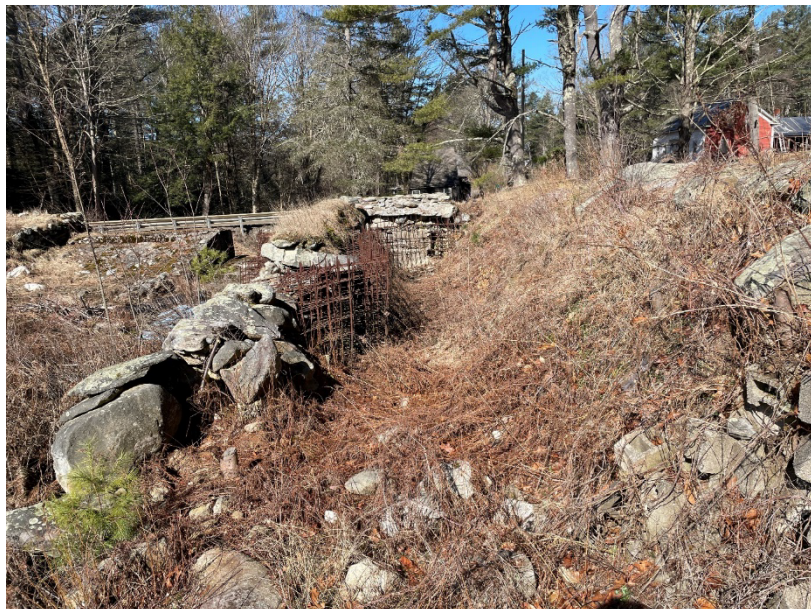
Photo 8. Overview of the excavated void space behind the right dam wall facing downstream
