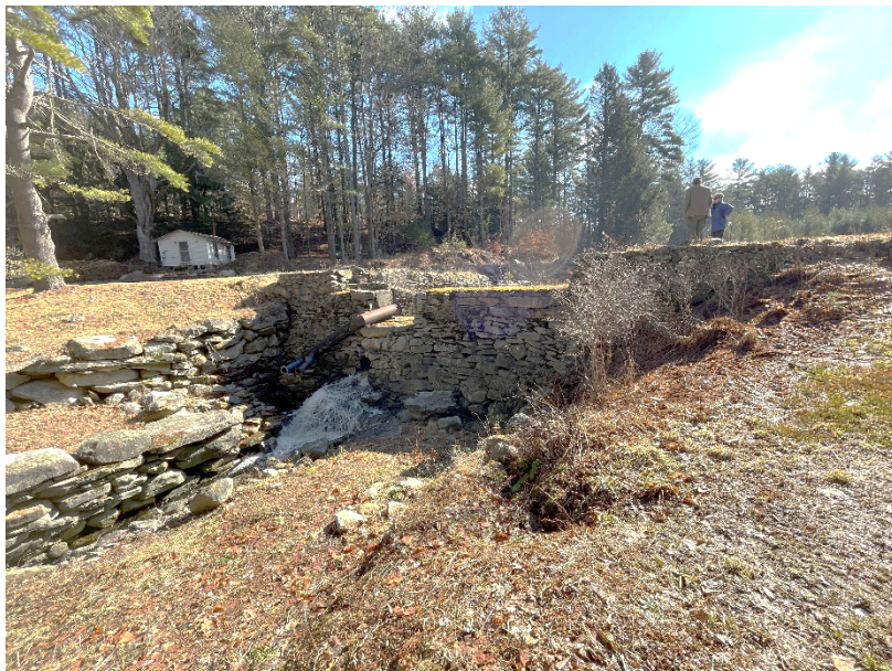
Photo 2. Overview of the dam facing upstream from the downstream left upper masonry wall
