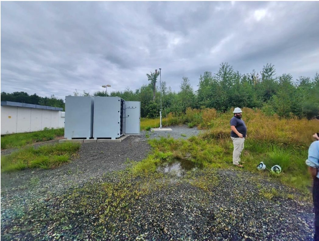
Location 5 (looking east). Northern lithium-ion battery pad showing the proximity of low vegetation to the battery cabinets and taller woody vegetation in the slope protection area in the background.
