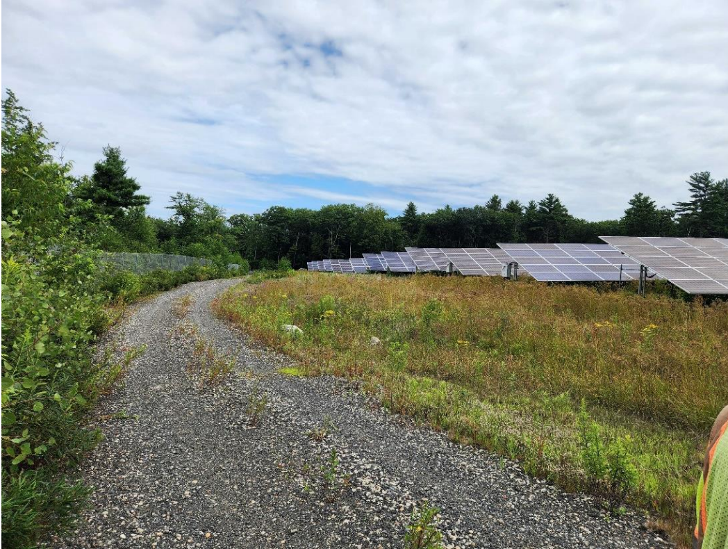
Location 4 (looking north). Service drive, western fence line, herbaceous ground cover, and western edge of arrays. The western stormwater detention pond (not visible) is located on the opposite side of the fence (left side of the photo).
