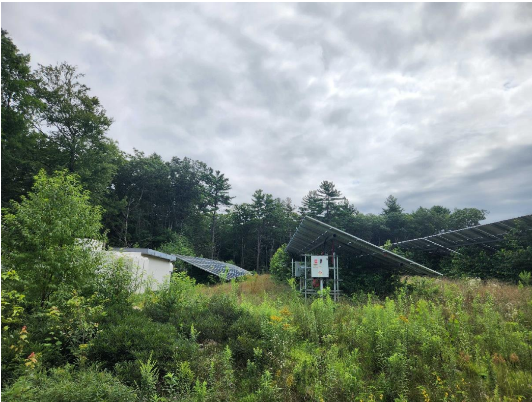
Location 3 (looking east). Herbaceous ground cover surrounding the solar arrays and electrical equipment.
