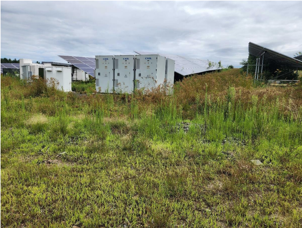
Location 6 (looking east). Southern lithium-ion battery pad showing the proximity of low vegetation around the battery cabinets.
