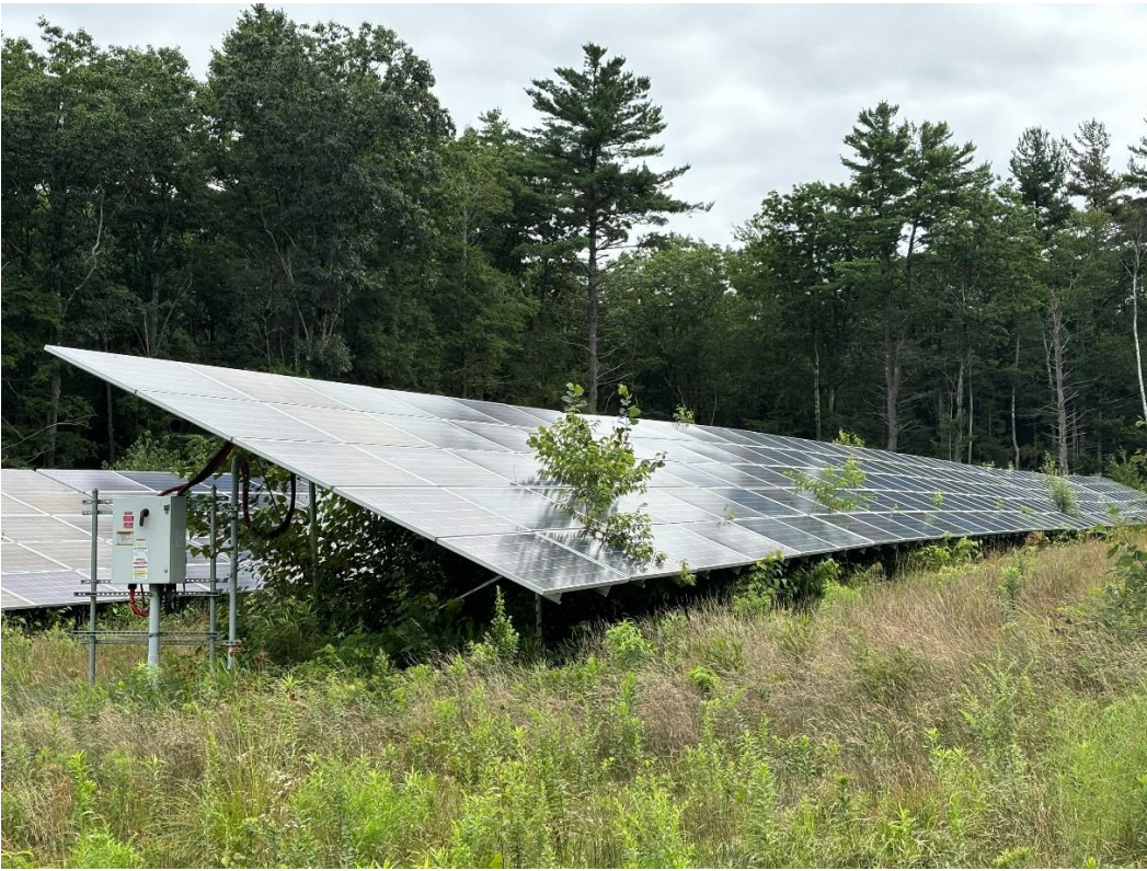
Location 3 (looking east). Herbaceous ground cover and woody vegetation growing up between solar panels.
