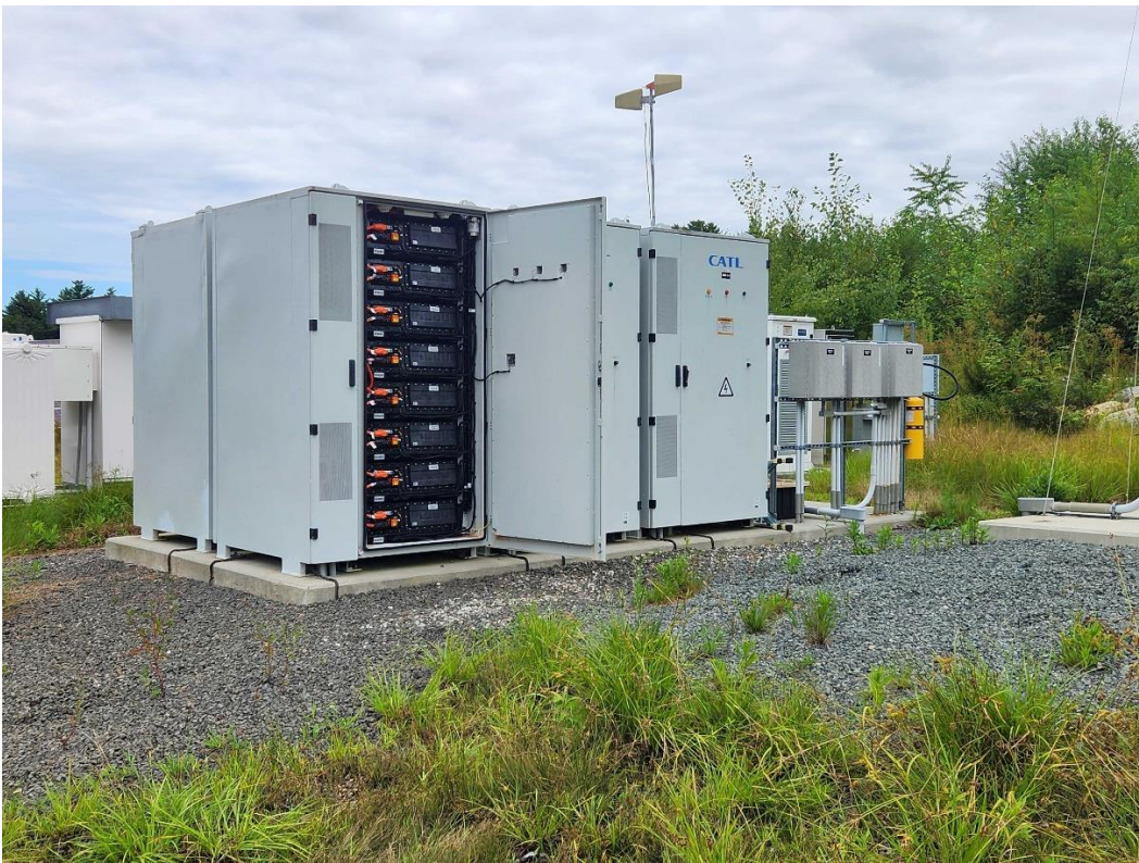
Location 5. Inside of a lithium-ion battery cabinet showing eight individual battery modules.
